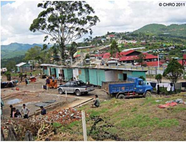
The civil servants working to clear the site of the Union Government guesthouse in Hakha, which is being rebuilt. The red building in the background is the Chin State parliament building, where Hung Ngai has his office. (Source: CHRO)
